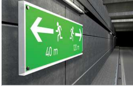
Emergency exit signs in tunnels
